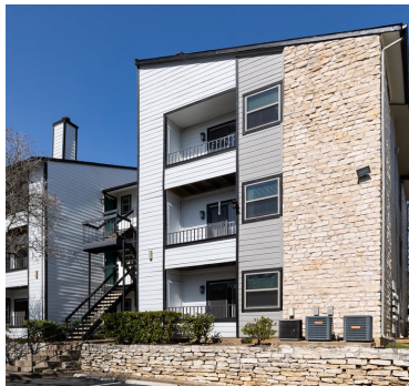
Contractors Inc performed extensive upgrades for Retreat at Barton Creek, an Austin, Texas, multifamily community with 20 buildings managed by Oden Hughes. The exterior renovations included siding, windows, painting, metal repairs, stone wall replacement and LED lighting. Image courtesy of Contractors Inc.
